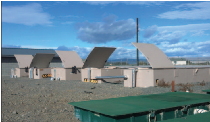
The Yakama Nations Housing Authority in Washington state added five AdvanTex® AX-Max units (background) to its ten AdvanTex AX-100 units, increasing the capacity of its wastewater system by 50%. Photo courtesy of Fextex Systems, Inc.
